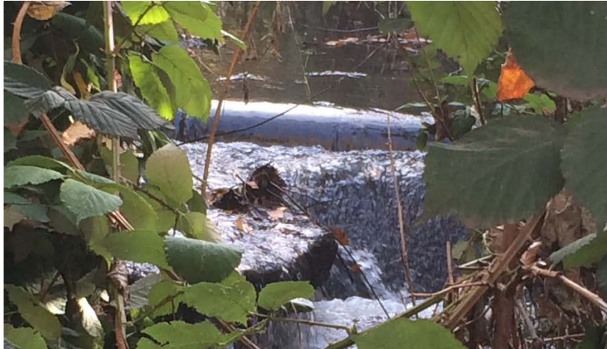
Exposed 12" water main near 35 th Street, Constructed 1958.
