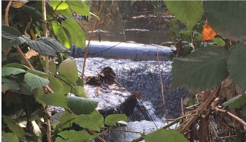
Exposed 12" water main near 35 th Street, Constructed 1958.
