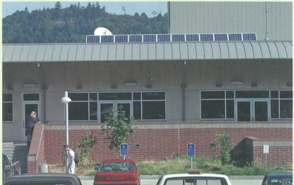
Solar photovoltaic panels generate electricity in Building 16, the math and science complex.
