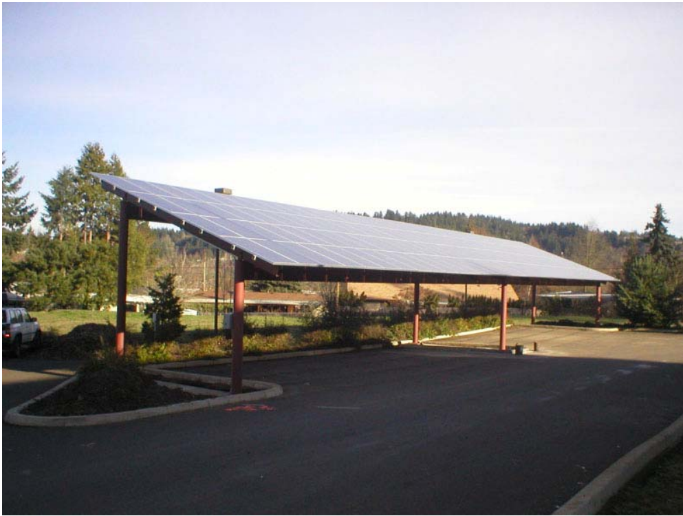
Example of a PV covered parking structure at the Tamarack Wellness Center in Eugene, OR.
