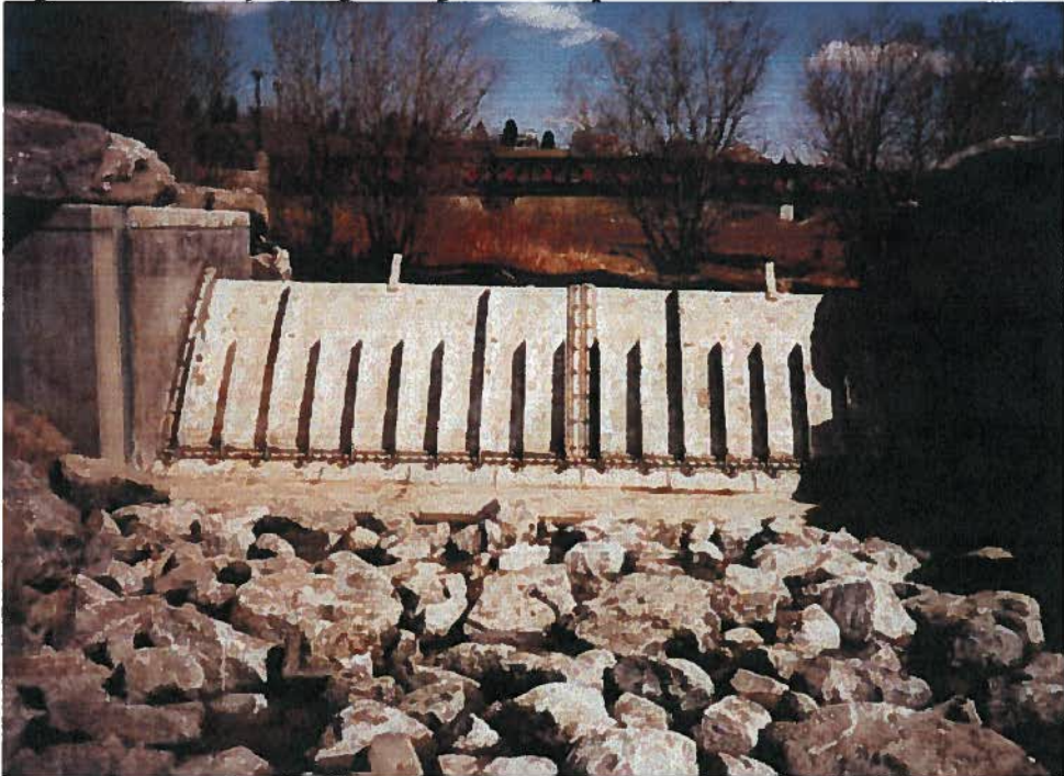
Figure 1 Obermeyer Regulating Weir – Upstream View
