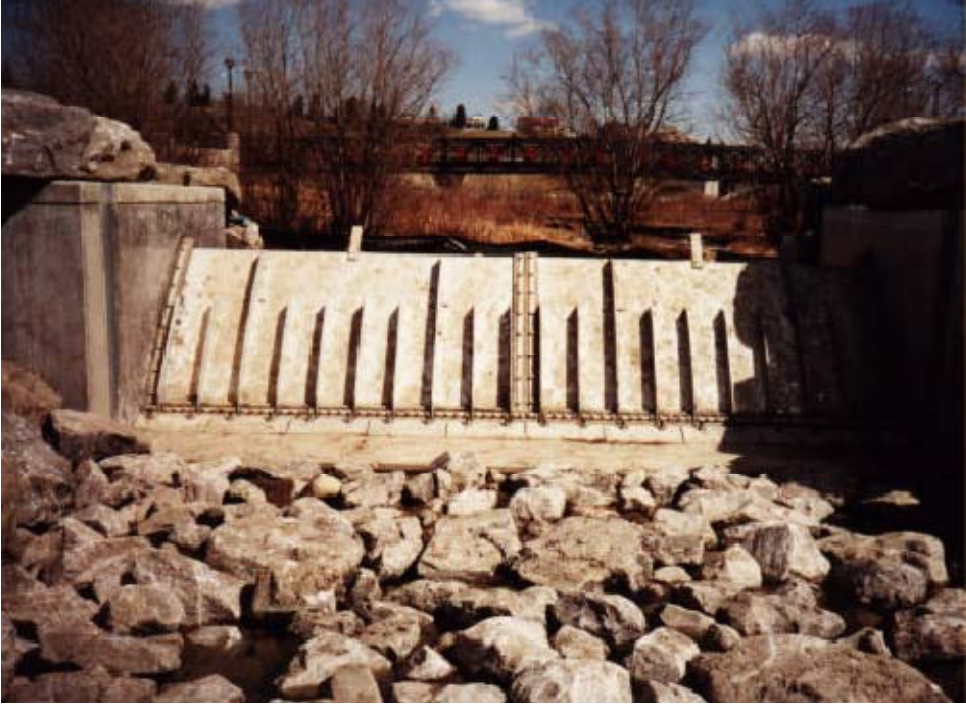
Figure 1 Obermeyer Regulating Weir – Upstream View
