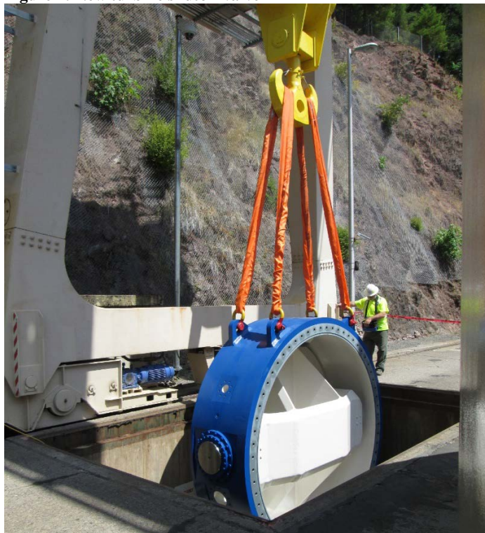
Figure 4: New turbine shutoff valve
